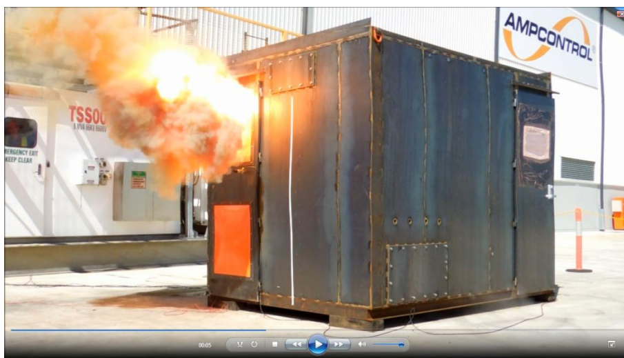
Figure 9: Arc vent rupture during simulated 30 kA fault.
