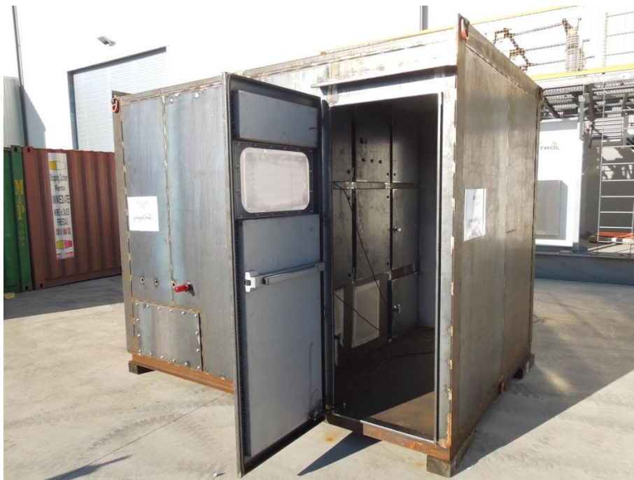
Figure 12: Control room end of mobile switchroom after simulated 30 KA fault.
