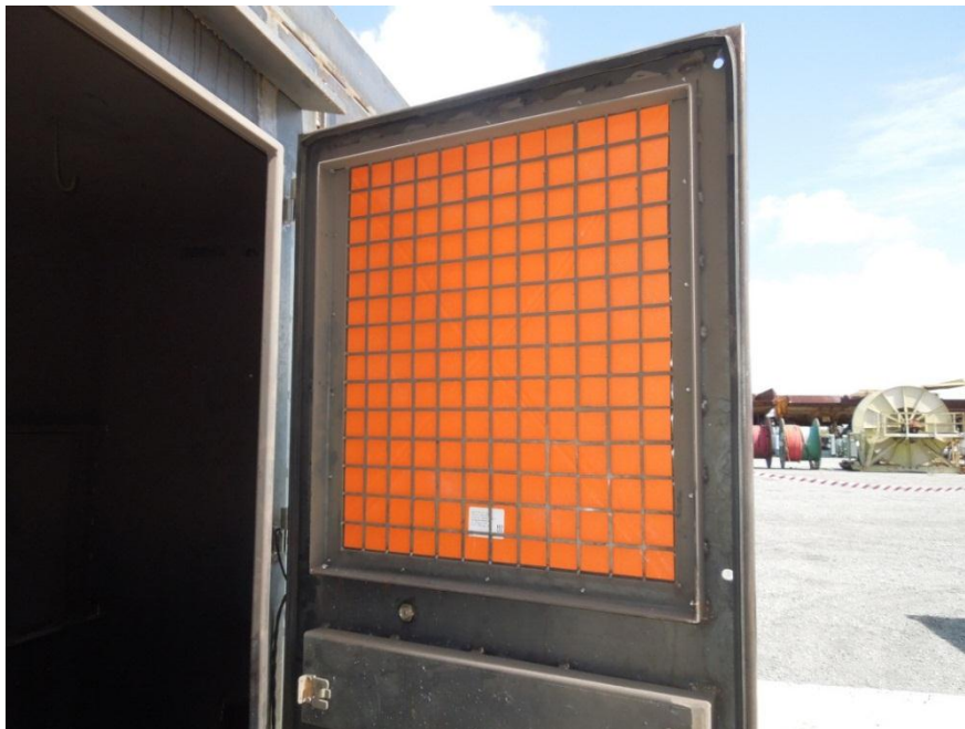
Figure 7: Amcontrol arc vent fitted to switchroom door.
