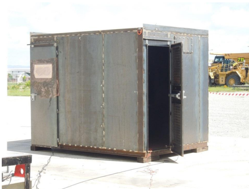
Figure 1: General configuration Ampcontrol Qld mobile switchroom.
